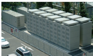
Installed NAS batteries
