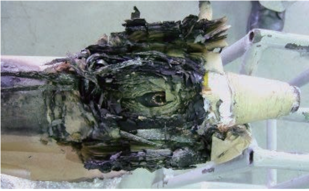
Figure 7 The Damage appearance of the cable core of the type A.
