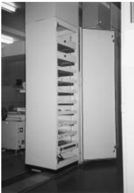
写真3 親局外観 Appearance of central equipment
