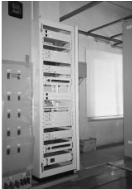
写真2 端局外観 Appearance of terminal equipment
