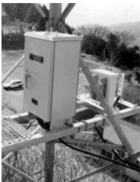
写真2 FL伝送局舎 Transmitter of fault location system
