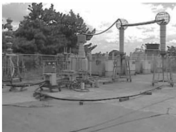
図10 66 kV CSJ長期化通電状況 66-kV CSJ long-term test
