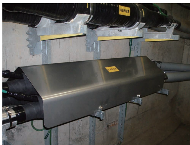
図4 ERJの現地据付状況(防護カバー設置後) View of assembled ERJ with protection cover.
