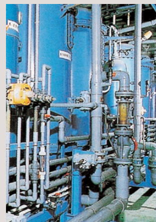
Wastewater treatment facilities
