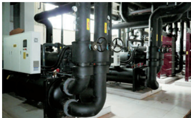
Switched from coal boilers to heat pump equipment for heating and preventing atmospheric pollution
