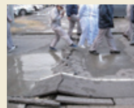
Road surface protrusion
