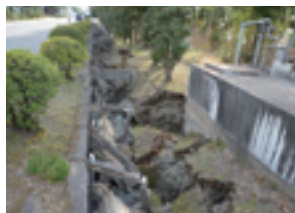
Broken central effluent pipe at the Chiba Works
