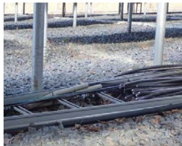
Disconnected CV cable
