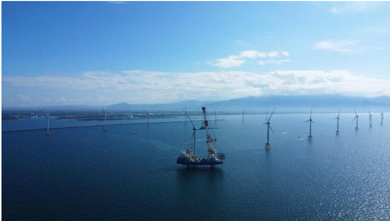
Ishikariwan Shinko offshore wind farm being installed (Picture provided by Green Power Investment Corporation)
