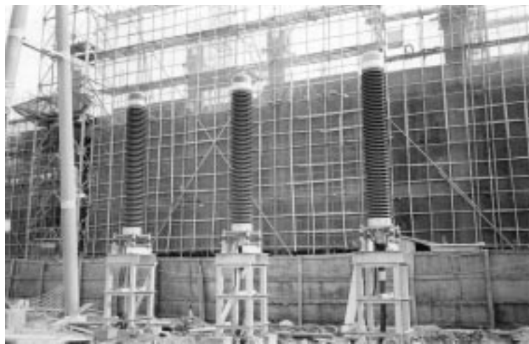
写真3 220 kV屋外端末の組み立て完成写真 View of completed 220-kV outdoor termination
