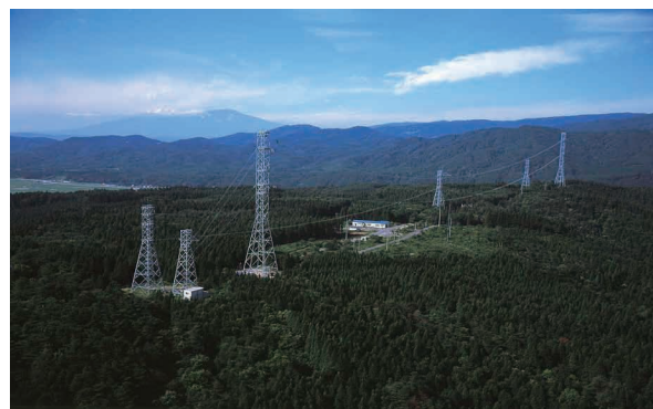
図33 最上試験線全景 Panoramic view of Mogami test line.
