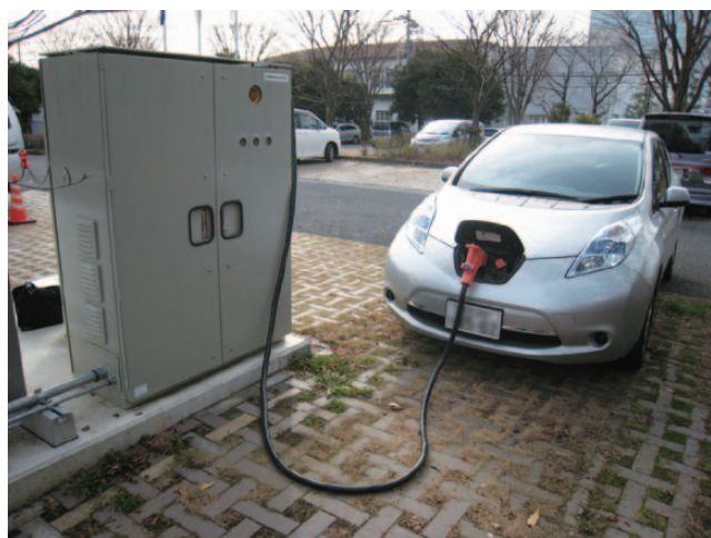
図4 EVとPCS Electric vehicle and power conditioning system.
