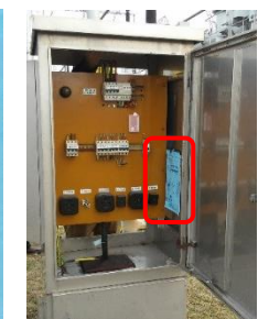
Inside an electrical box
